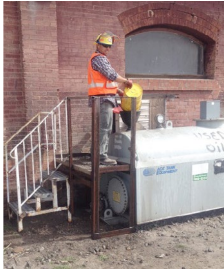
After: Fernando Zavala, machine operator, easily empties oil into the container thanks to the new steps and deck constructed by the Ogden, Utah, TSC I-Team.
