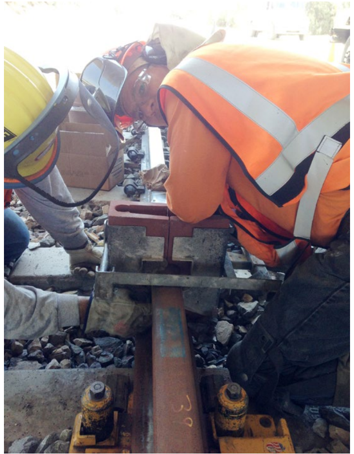
Members of the Phoenix Maintenance of Way crew begin a thermite weld. From left are Rafael Garcia and Robert Long.
